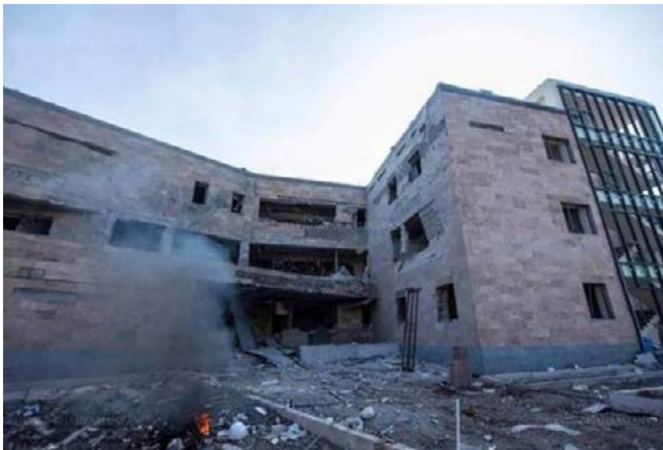
Figure 15.11. Damage to the Stepanakert Maternity Hospital, 28 October 2020 (Source: Massis Post).
