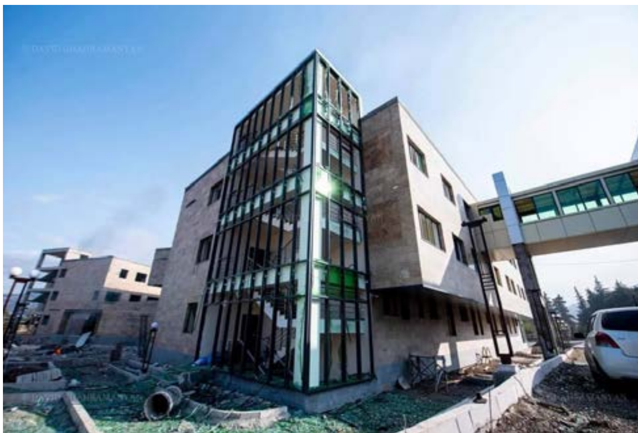
Figure 15.12. Damage to the Stepanakert Maternity Hospital, 28 October 2020 (source: Massis Post, 2020).
