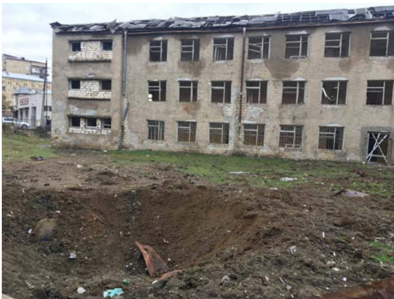
Figure 15.45. Damage from a munition which exploded near School No. 10, 2020 (Source: Fact-Finding Group).
