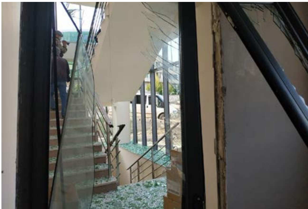
Figure 15.15. Damage to the Stepanakert Maternity Hospital, 28 October 2020 (Source: Infoteka24).
