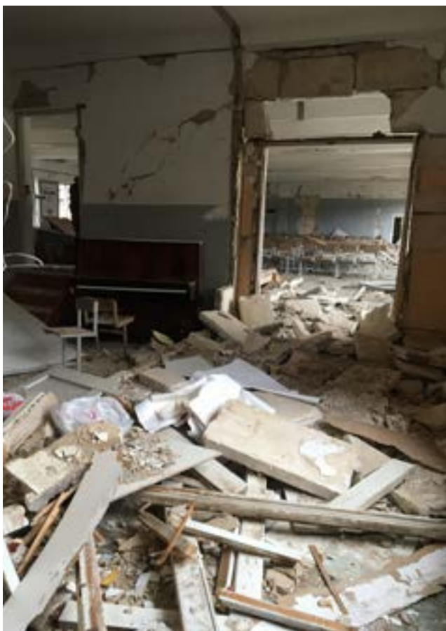
Figure 15.47. Damage from a munition which exploded near School No. 10, 2020 (Source: Fact-Finding Group).
