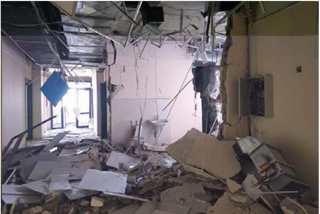
Figure 15.14. Damage to the Stepanakert Maternity Hospital, 28 October 2020 (Source: Panarmenian.net).
