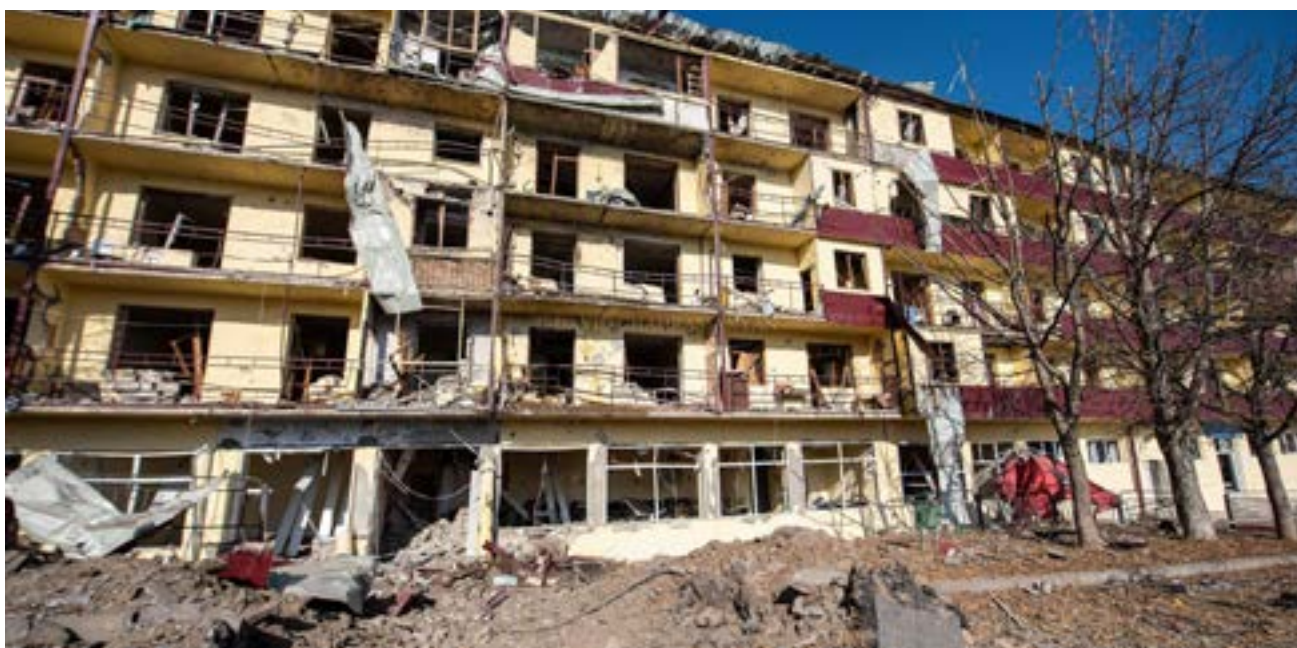
Figure 15.63. Building on Ghazanchetsots street after shelling, 29 October 2020 (Source: MFA Armenia).
