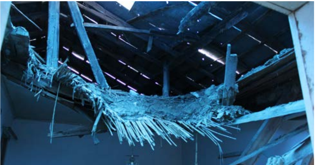
Figure 7.38. Damaged roof of N.B.'s house, Martuni city, 11 December 2020 (Source: Fact-Finding Group).
