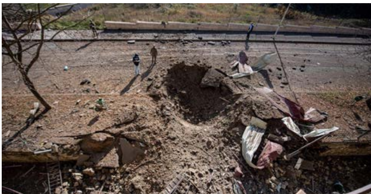
Figure 15.64. Crater near the building entrance created by shelling, 29 October 2020 (Source: MFA Armenia).
