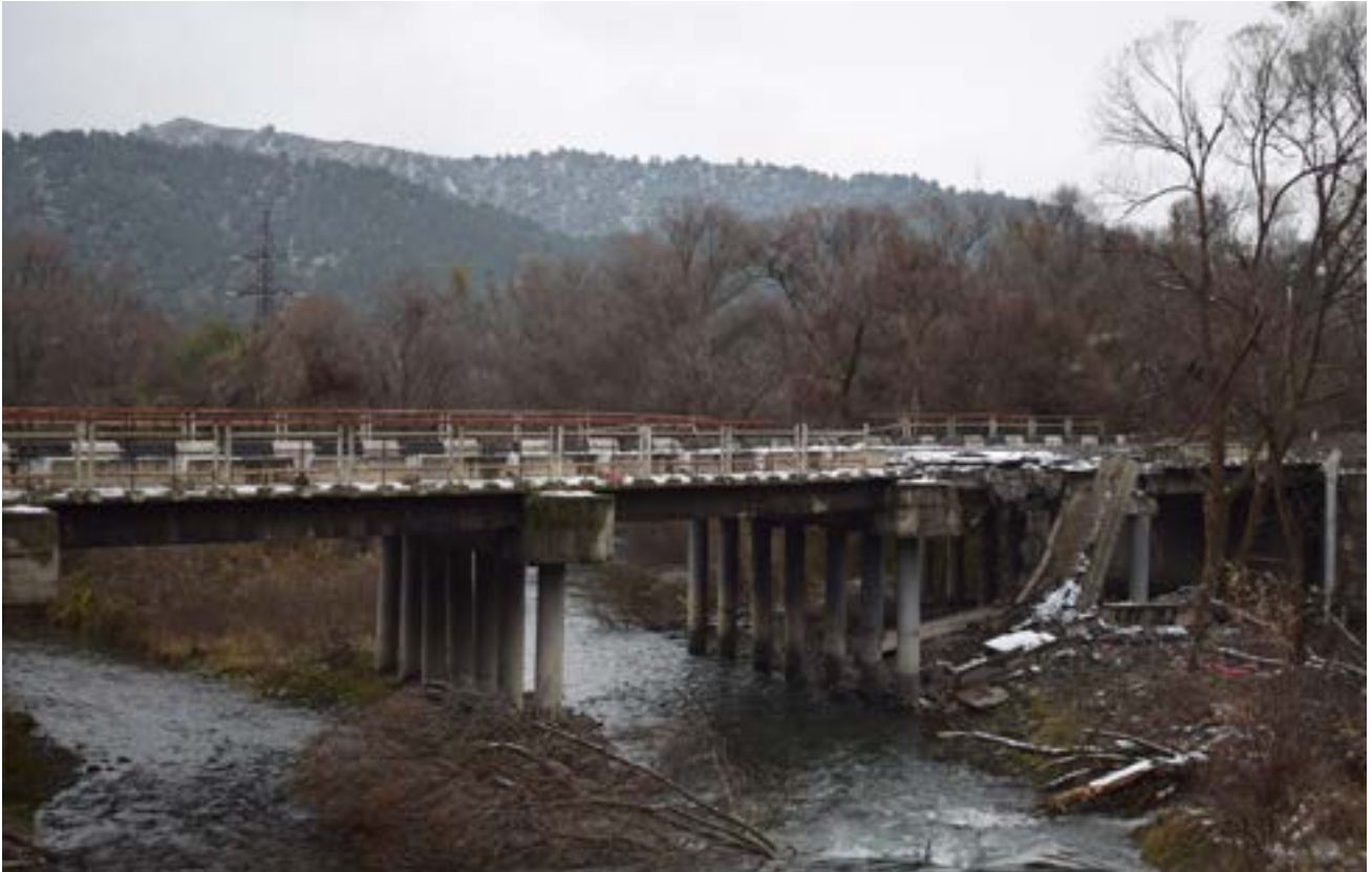
Figure 15. 21. Damage to the Berdzor bridge, 2 October 2020 (Source: Fact-Finding Group).
