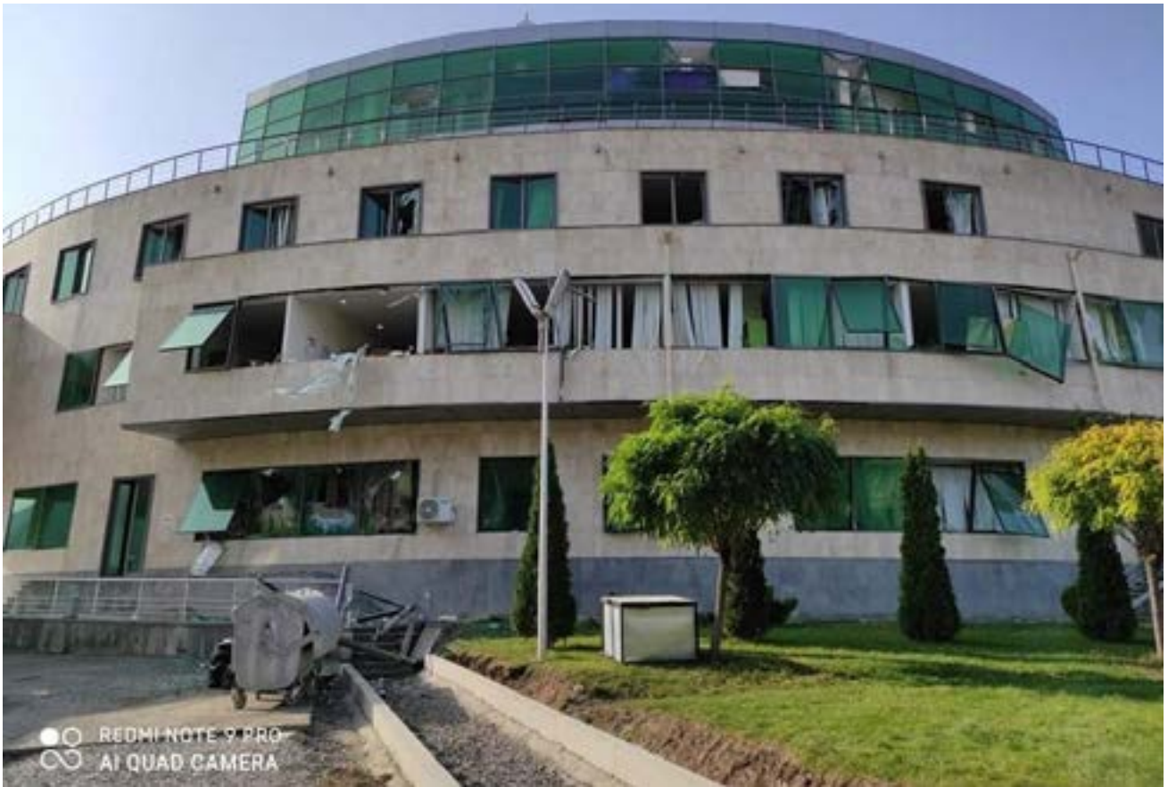
Figure 15.13. Damage to the Stepanakert Maternity Hospital, 28 October 2020 (Source: Tigran Mkrtychyan's Twitter account (@TMkrtychyan)).
