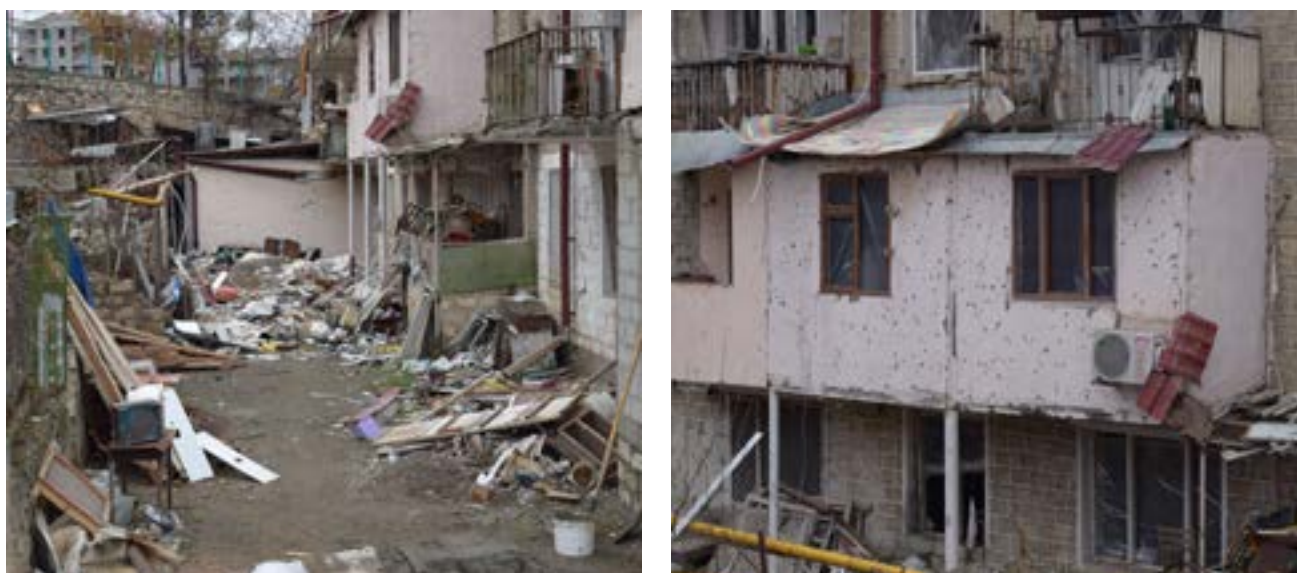
Figure 7.42. Pictures of the targeted buildings at Alek Manukyan Street, Stepanakert city, 12 December 2020 (Source: Fact-Finding Group).
