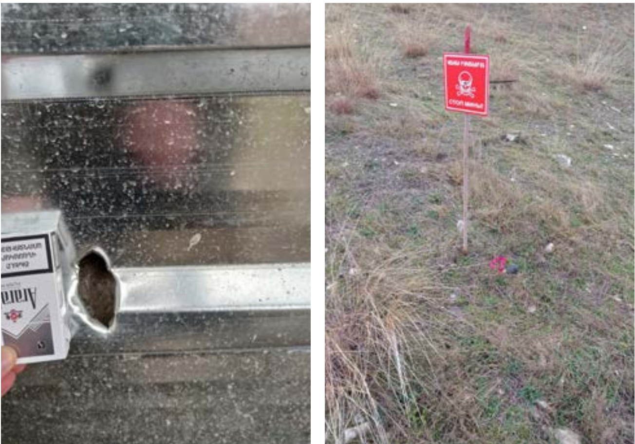
Figure 15.71. Damaged wall of Shahen Balayan's house after the attack that killed his wife and a submunition found in the yard of Shahen Balayan's house, 2020 (Source: Fact Finding Group).
