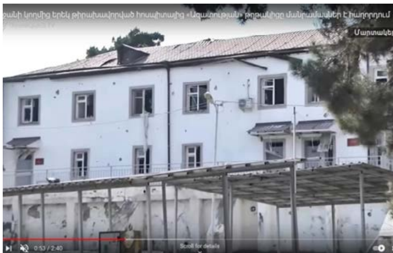
Figure 15.6. Fragmentation damage to the main building of the Martakert's Military Hospital, 14 October 2020. (Source: «Azatutyun» TV).
