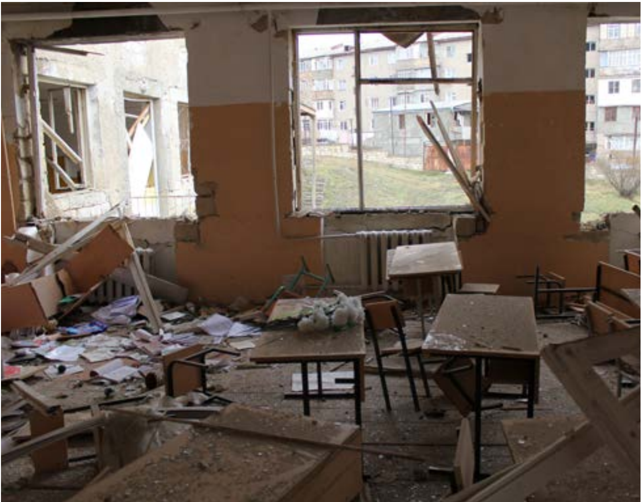
Figure 15.46. Damage from a munition which exploded near School No. 10, 2020 (Source: Fact-Finding Group).
