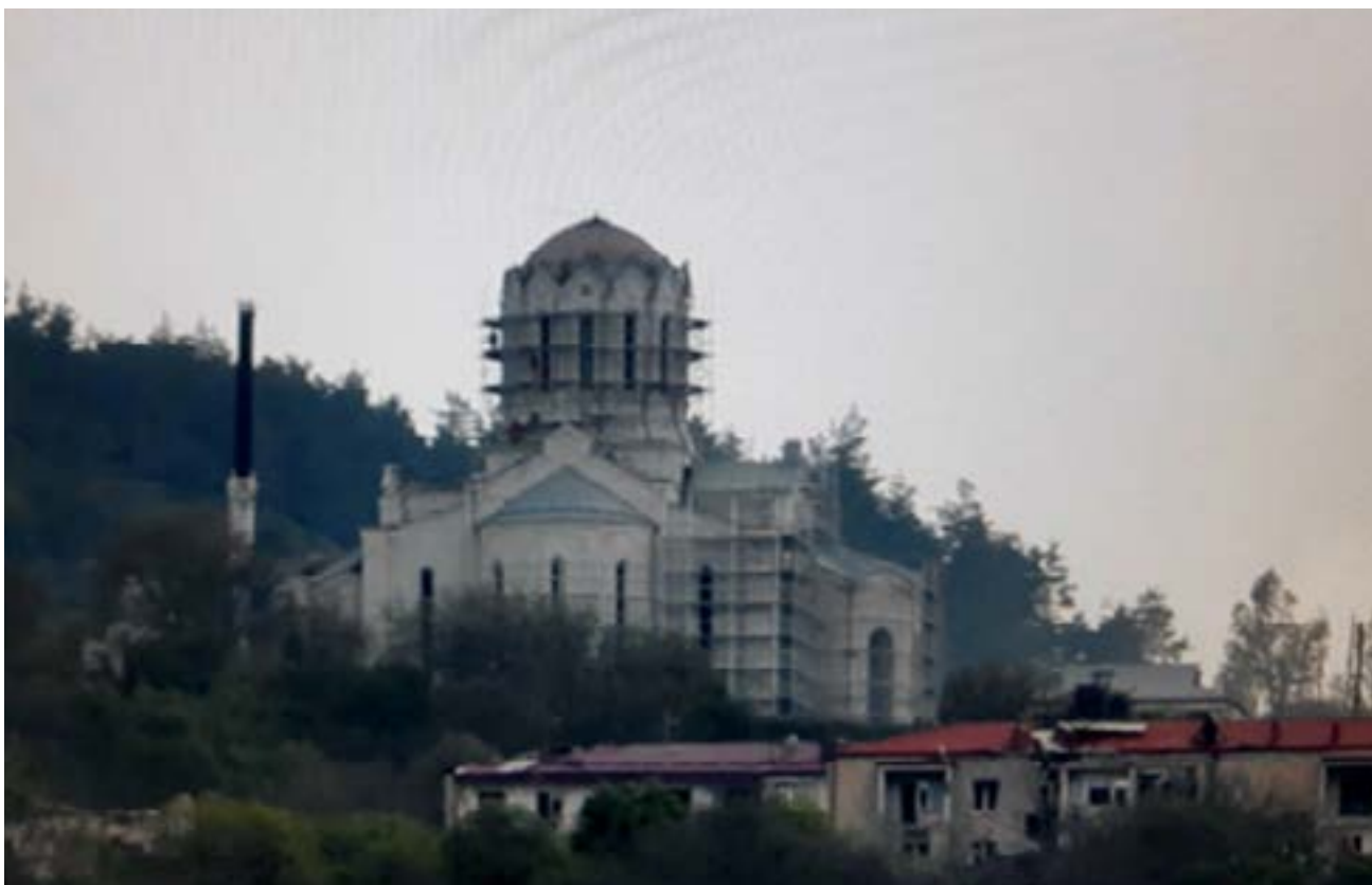
Figure 13.9. The Azerbaijani side carrying out structural works to change the architectural appearance of the Ghazanchetsots Cathedral, 03 May 2021 (Source: Public Radio Armenia).
