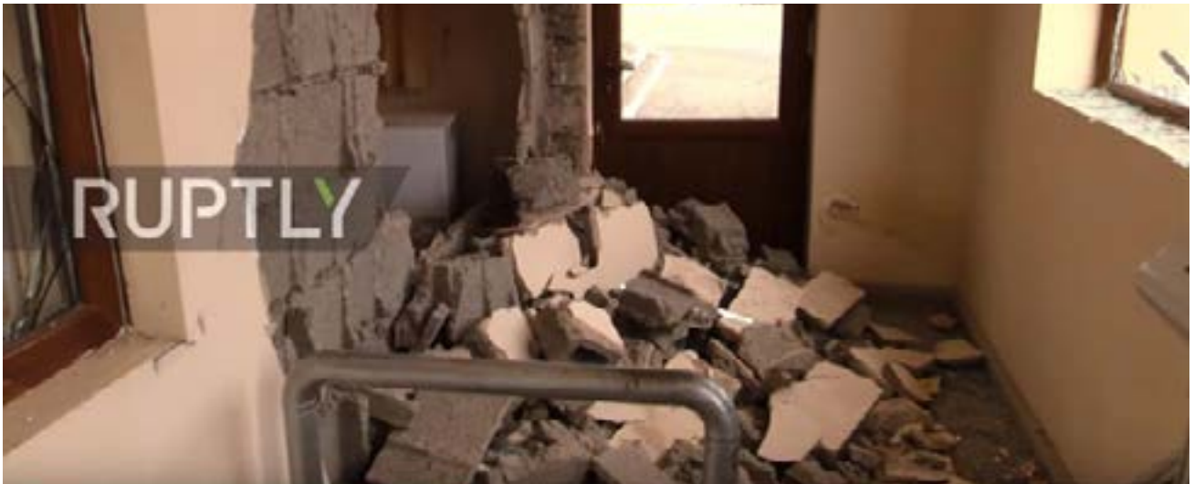
Figure 15.16. Internal structural damage likely caused by blast overpressure on the exterior gatehouse outside the main building of the Rescue Service of Artsakh, 2020 (source: Ruptly).
