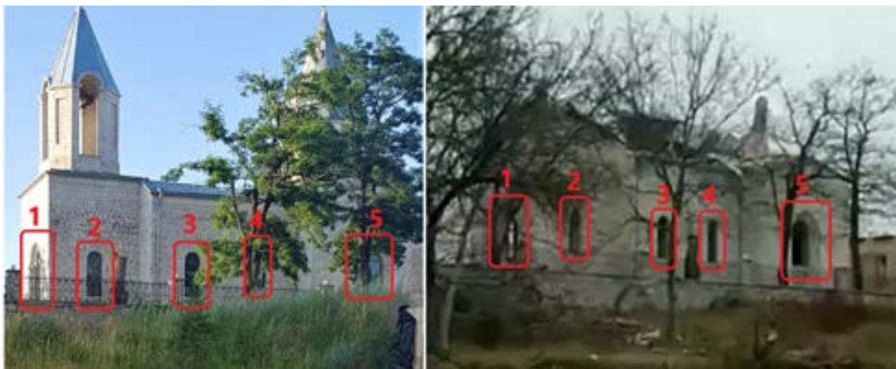
Figure 13.10. St. John the Baptist (Kanach Zham) church before and after destruction, 2020 (Source: Fact Investigation Platform).
