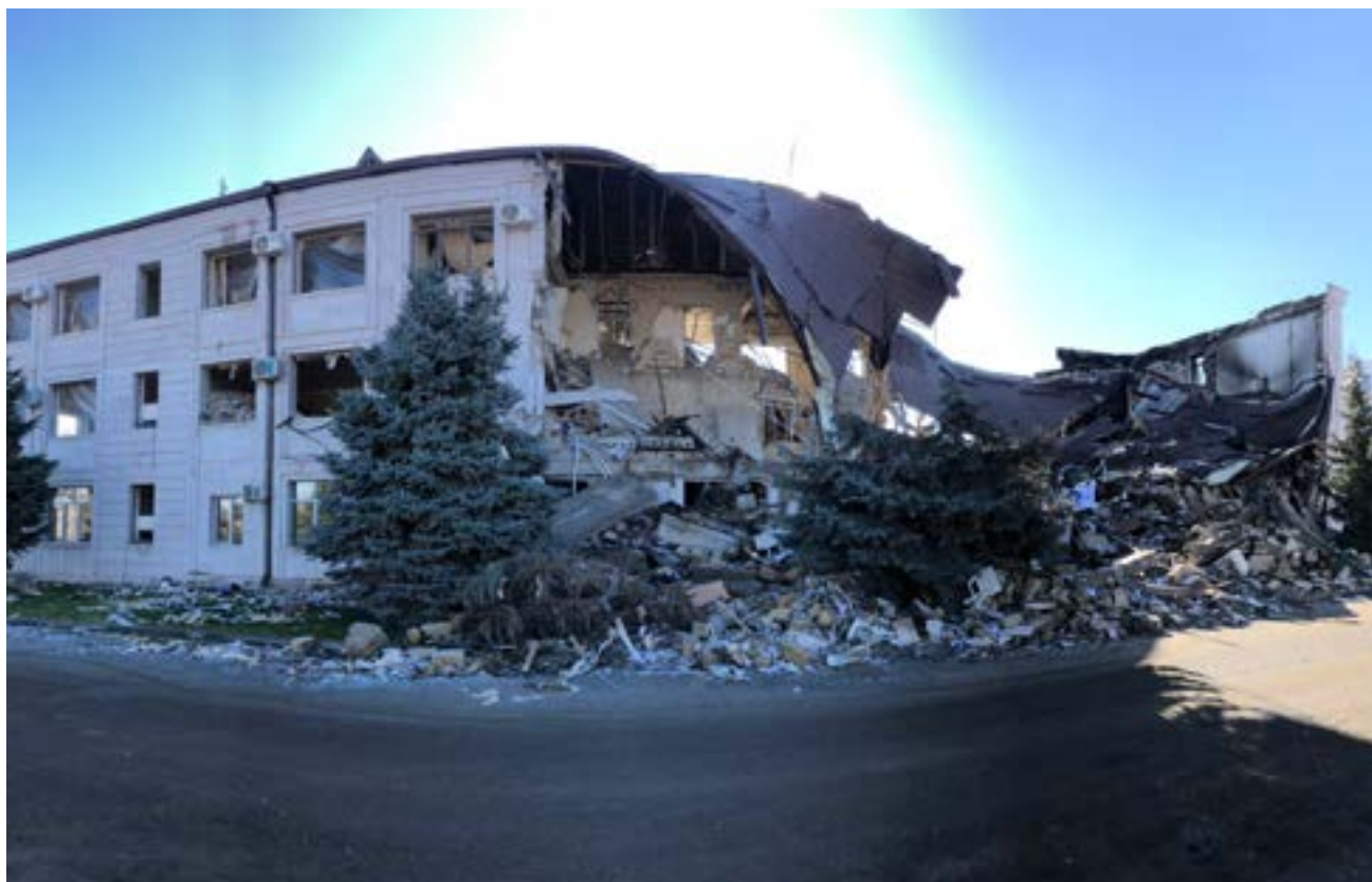
Figure 15.19. The badly damaged Administrative Building of “Artsakhenergo” in Stepanakert after an attack, 4 October 2020, showing structural collapse typical to buildings damaged by one or more large blasts (source: Fact-Finding Group).
