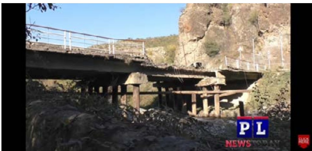
Figure 15. 20. Damage to the Aghavno checkpoint bridge, 17 October 2020 (Source: Patric Lancaster's Youtube Channel).
