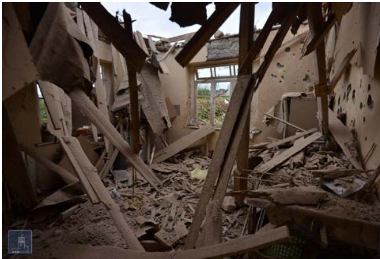
Figure 15.68. Documented damage to the interior of the building next to which was found part of the munition body ('casing') of an Israeli Elbit Systems LAR-160 surface-to-surface rocket, 27 September 2020 (Source: MFA Armenia).
